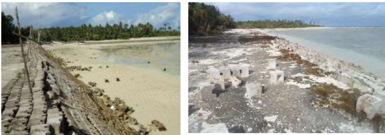
Figure 7 Block seawall in Nukufetau before (left) and after (right) Cyclone Pam
